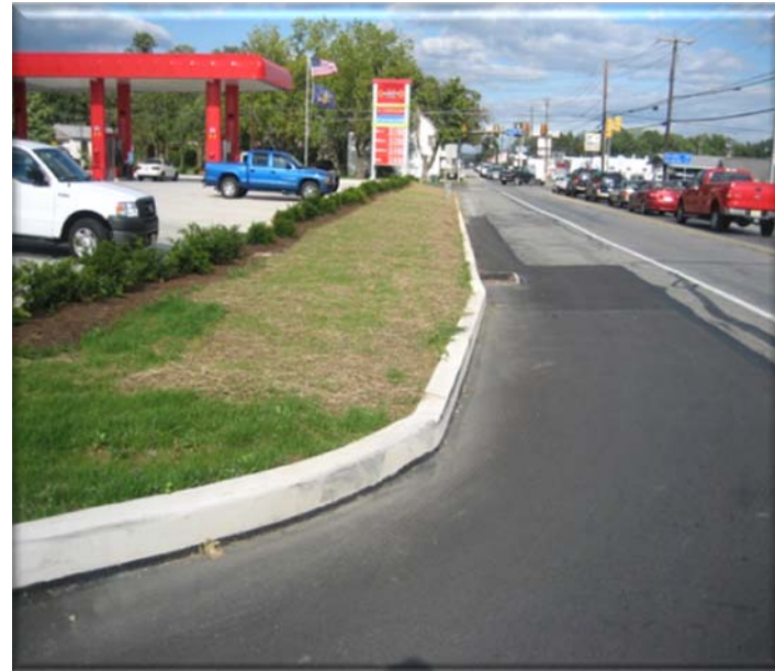
Existing Manhole converted to Inlet which is part of an existing system
