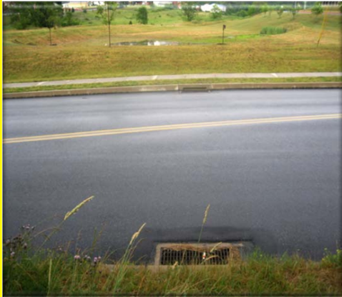
Detention Basin draining into existing Department cross-pipe
